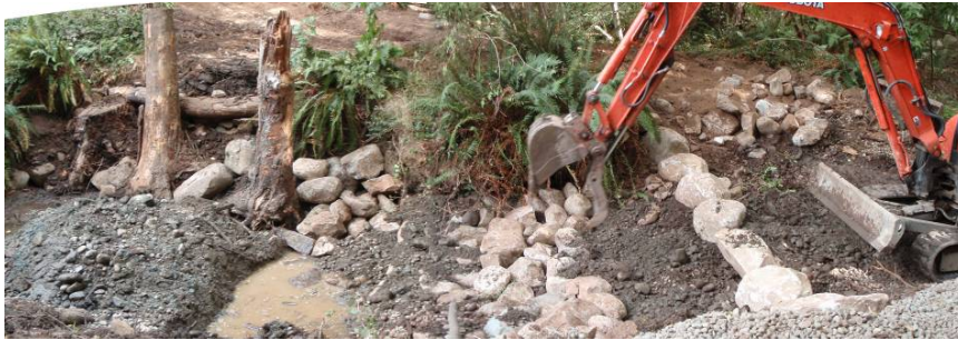
Photo 2 & 3. Installation of riffle and LWD features at km 1+200 during (top) and after construction (bottom) on Aug 19 & Oct 14 respectively.
