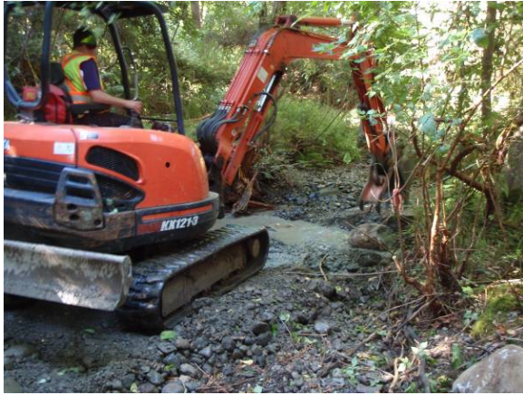
Photo 1. Construction of rock riffle using small excavator positioned in stream channel. (Aug 24, 2010).
