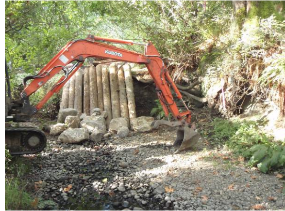
Photo 8. Temporary bank protection using logs to reduce impact of boulders delivered by bobcat to riffle construction site (Aug 17, 2010).
